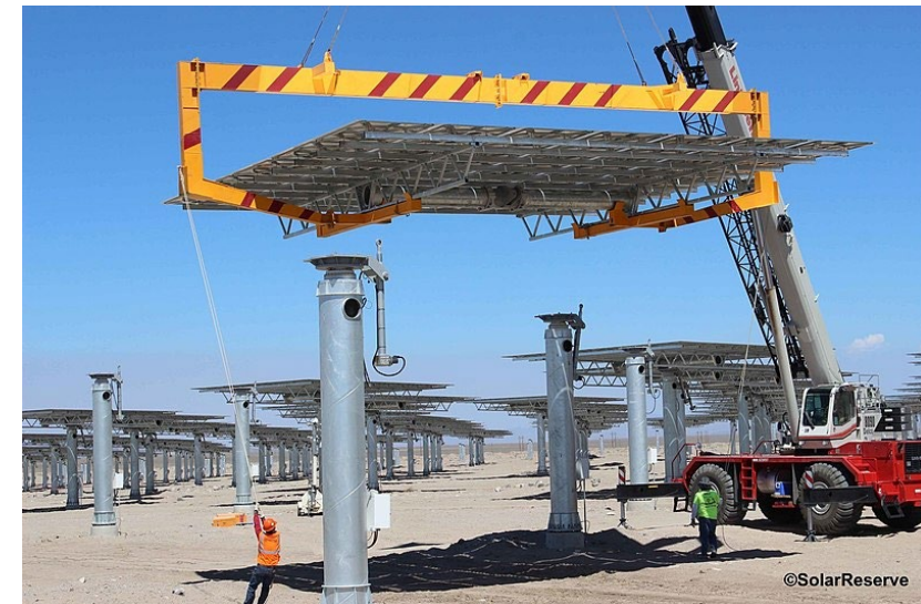
A heliostat is crane-lifted onto a pylon. Typically, no shape validation is done after this is complete.
